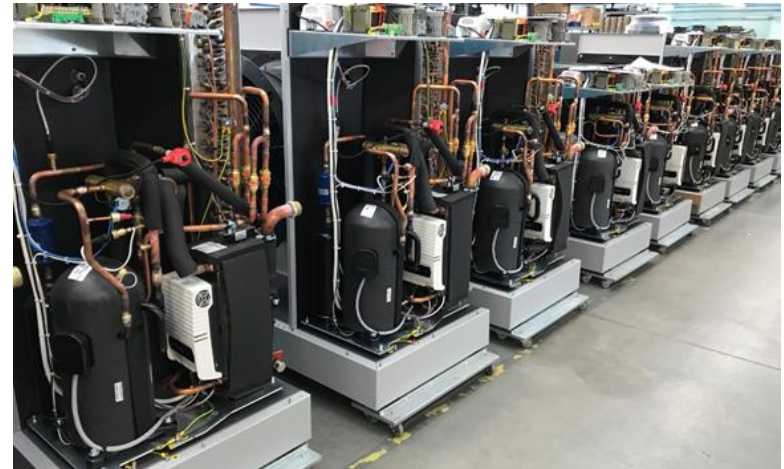
Batch production plant Dobré
